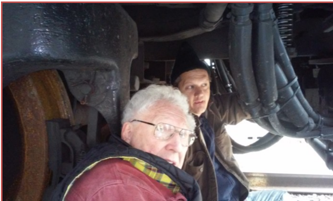
Paul Flanagan (l) and Jim Lilly (r) under the A-end of the Dover Harbor at Dover Park, working on the coupler carrier iron. Some jobs require the members of the mechanical committee to get a bit dirty! Photo by John Zabrosky.
